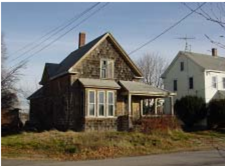
Boarded-up house, Stoughton
